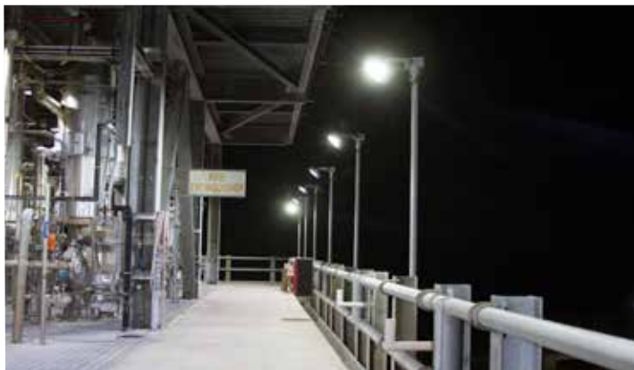
Dialight SafeSite Area Lights were an easy install.
