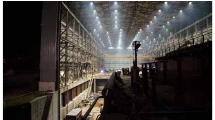
After: Dialight Vigilant 60,000lm High Bay Fixtures at Donjon
