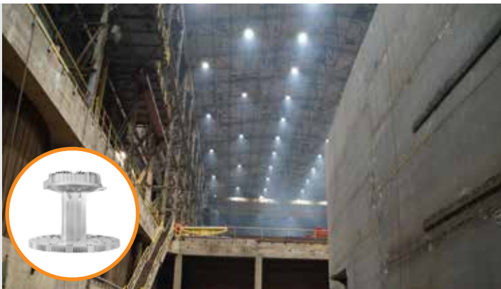
Dialight Vigilant® 60,000lm LED High Bay Fixtures cut through the dust at Donjon Shipbuilding and Repair
